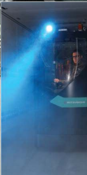
Pedestrian warning system
